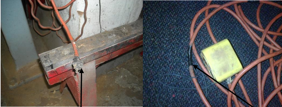
Missing ground pin
