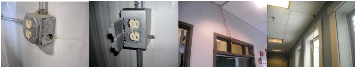
Damaged Junction Box; Damaged Cover plate. Flexible cords through window and ceiling tiles.
