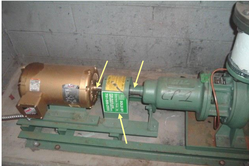
An inadequate guard on a small heating system pump. The shaft is exposed on both the motor and pump sides of the coupling.
